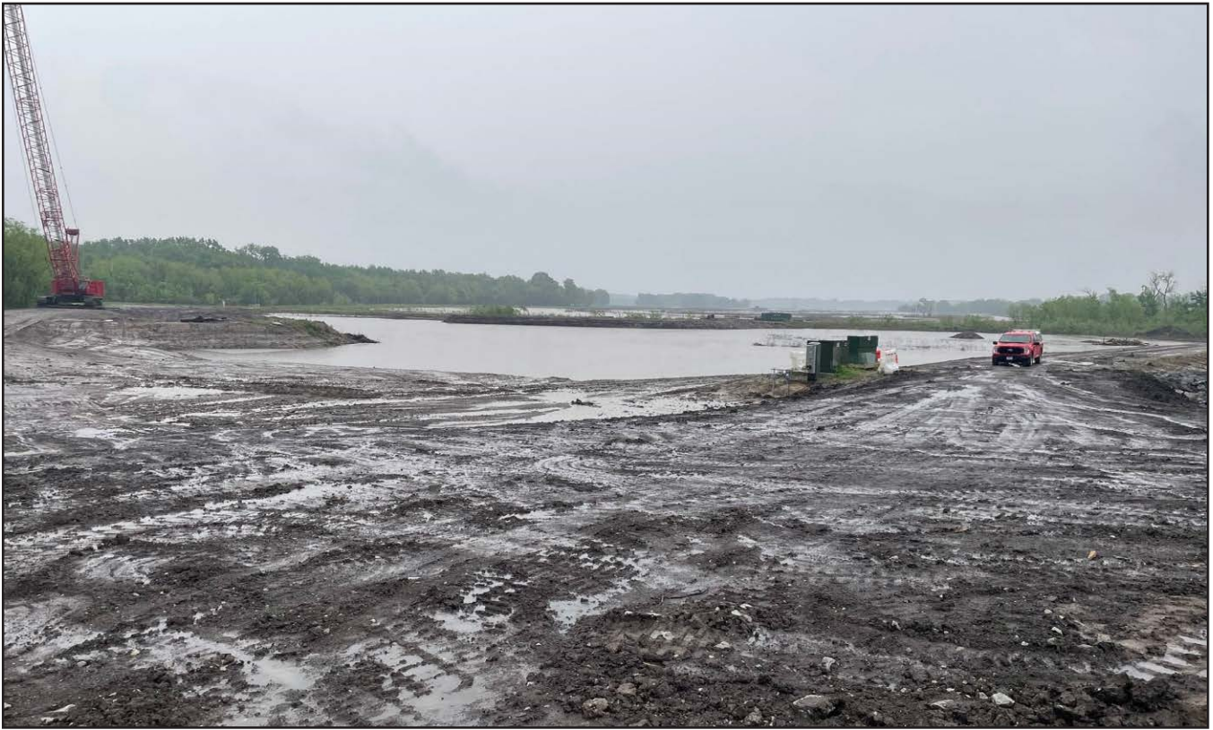
The construction site at Fountain Grove in April as it was impacted by rain and a rising Grand River.
